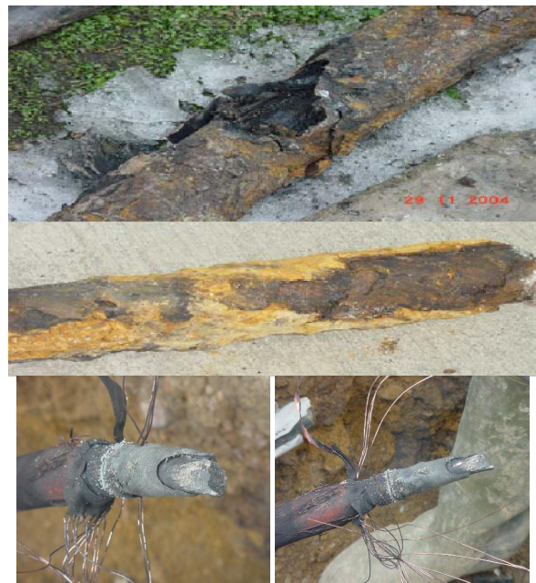
Figure 18. Advanced corrosion of a medium voltage cable in Cluj, due to stray currents caused by trams [24]
