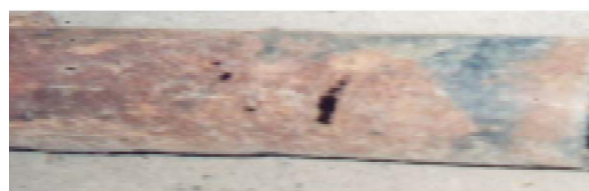
Figure 21. Generalized corrosion caused by composed (D.C.+A.C.) stray currents
