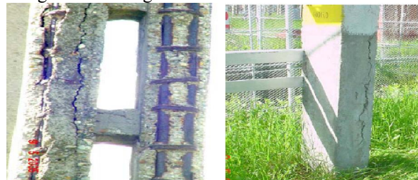
Figure 20. Steel concrete support elements (operating in high level electromagnetic field) degradations [22]
