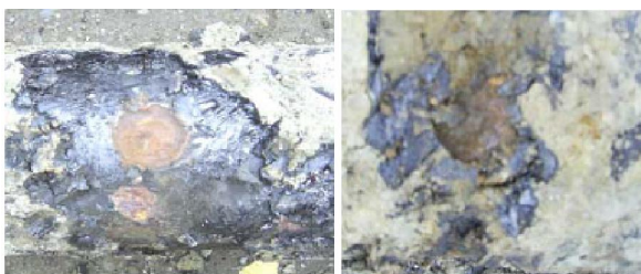
Figure 17. Localized corrosion on some gas pipes due to D.C. stray currents of trams and underground train in Bucharest
