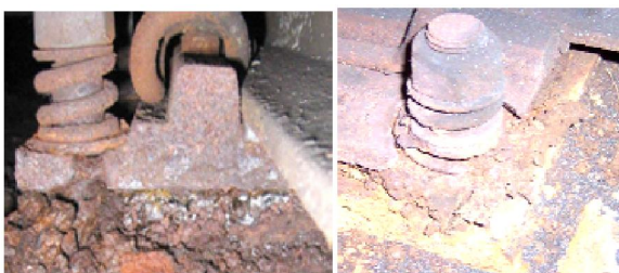
Figure 16. Advanced damages fixing element at underground train in Budapest (formed in about 2 years) due to D.C. stray currents
