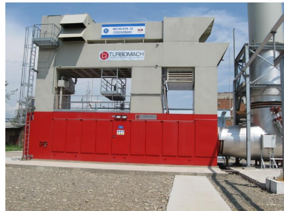
Fig. 3. Natural gas fired cogeneration unit: the gas turbine ( http://www.free.org.ro )
