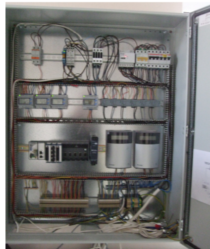
Fig. 13 – The control box
