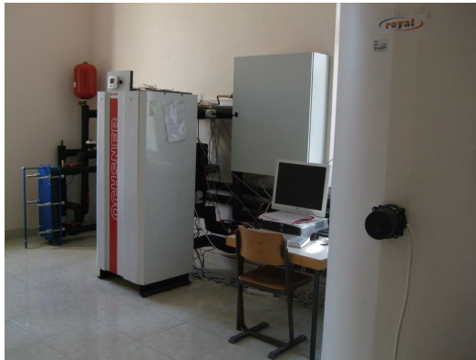
Fig. 12 – The technical room
