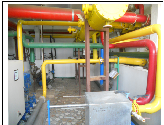
Fig. 4. Geothermal main station Operating in Nufarul district
