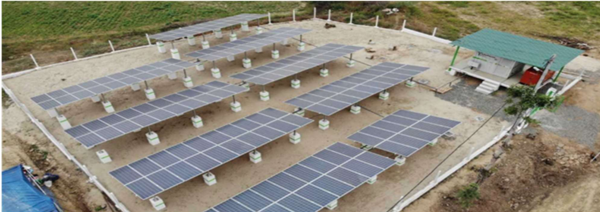
Fig. 14. 100 kW solar photovoltaic mini-grid in Akpabom Community, Onna LGA., Akwa Ibom, Nigeria, being managed by GVE
