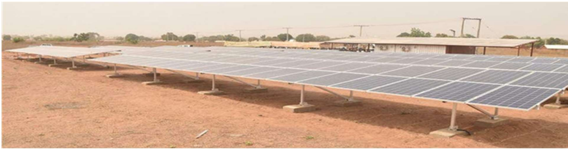
Fig. 13. 157 kW capacity solar photovoltaic power plant at Rokota, a community in Niger State, Nigeria
